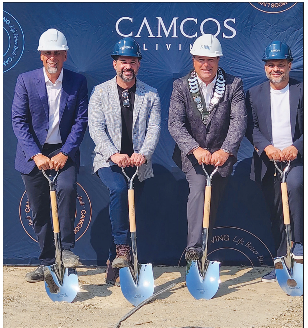
The shovels went in the ground last week to launch the King City condo project by Camcos. Shown are (l to r) James Circosta, Mike Circosta, Mayor Steve Pellegrini and Nino Campoli.
