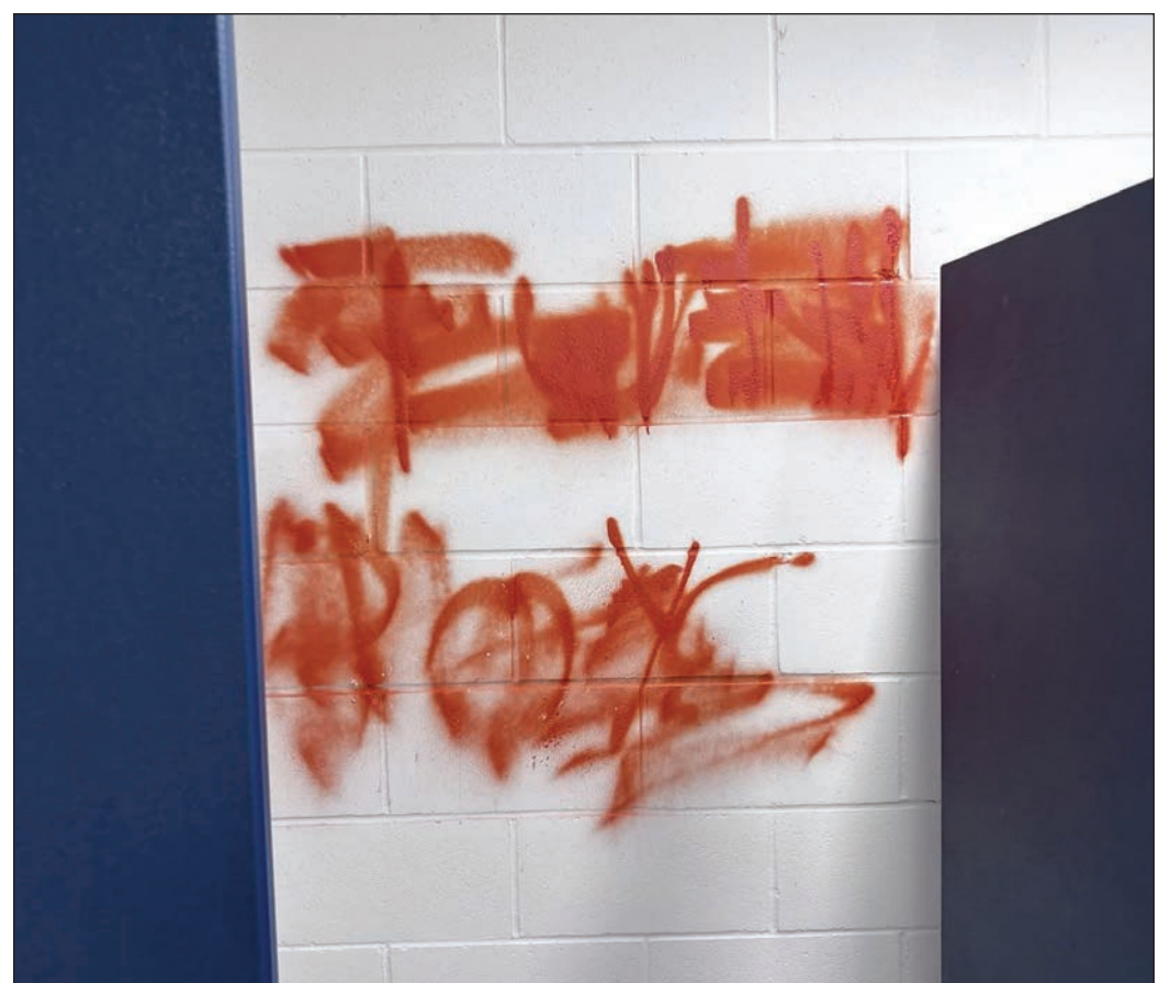
Vandalism curtails washroom hours at park
