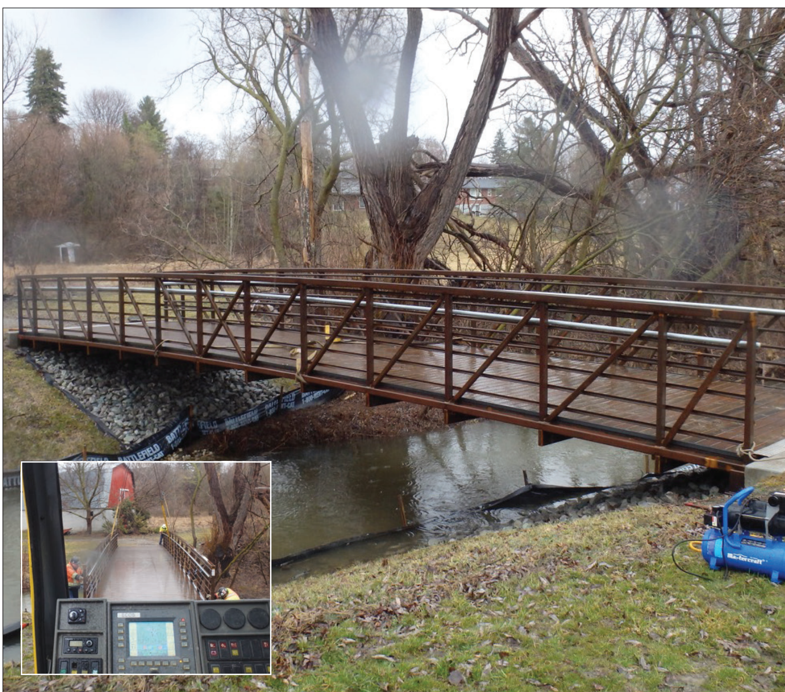
The long-awaited bridge that now connects the Schomberg Community Farm was installed April 4, is a welcome addition to the community.
