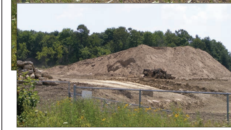
King Township's newest park is taking shape. Many features are planned for the 21-acre park in Nobleton. Photos by Mark Pavilons
