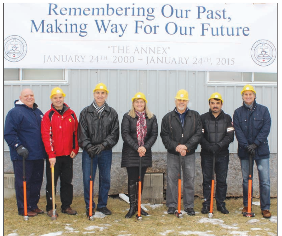
As one chapter of Villanova College’s history came to a close, another one begins. The original portable was demolished Saturday, making way for future plans for continued growth at the campus.
