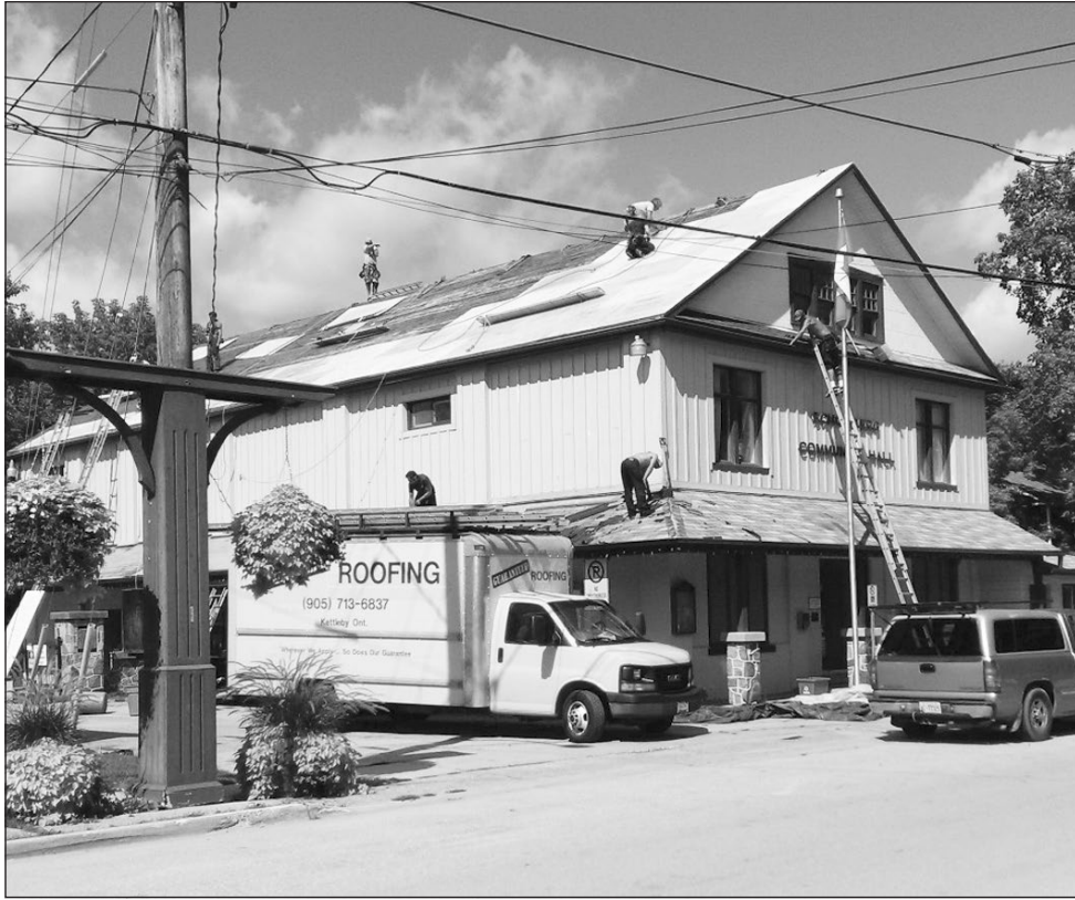
The Schomberg Community Hall got a new roof! The crew made quick work of the project over a couple of days and the result looks great.
